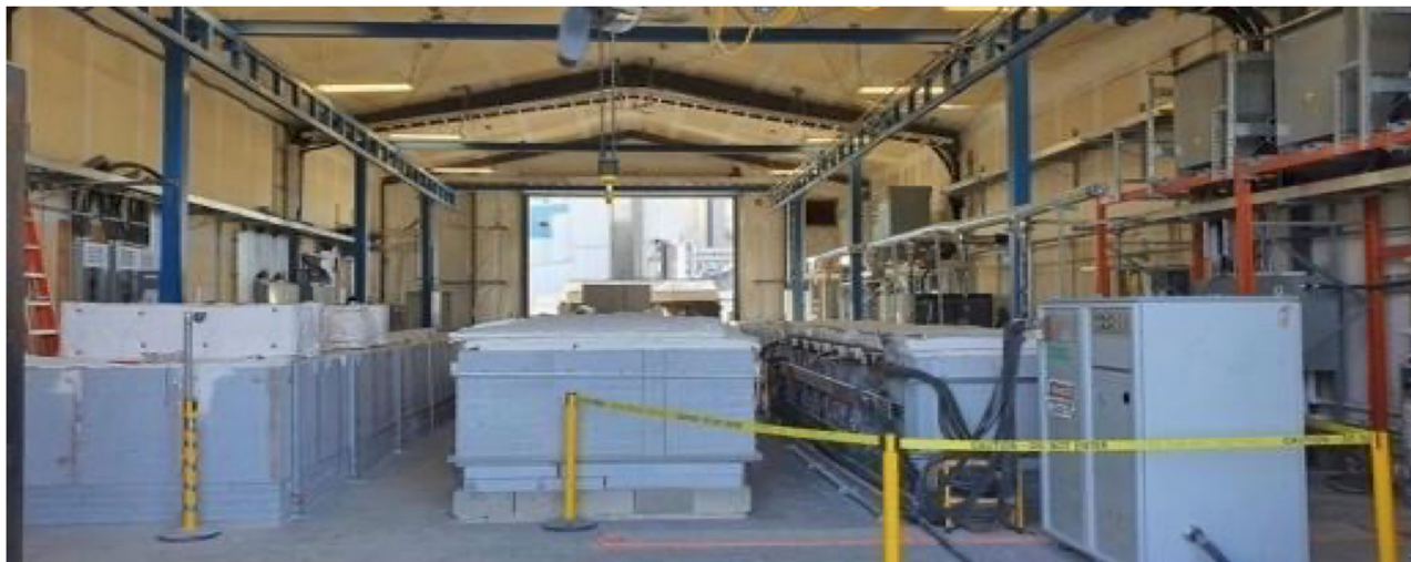
Fig. 14 | The Genesis Device ® kiln used for large-scale CO 2 molten carbonate electrolysis. The decarbonization kilns are onsite at Carbon Corp in Calgary, Canada.
