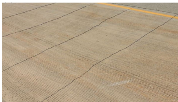
Figure 5. Straight crack propagation from saw-cuts in the CRCP section 18 .
