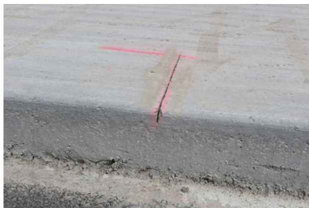
Figure 4. Early entry partial surface saw cut made in the CRCP slab in Illinois, United States 18 .
