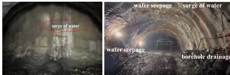
Fig. 5. (a) Surging water. (b) Seepage and surge water.
