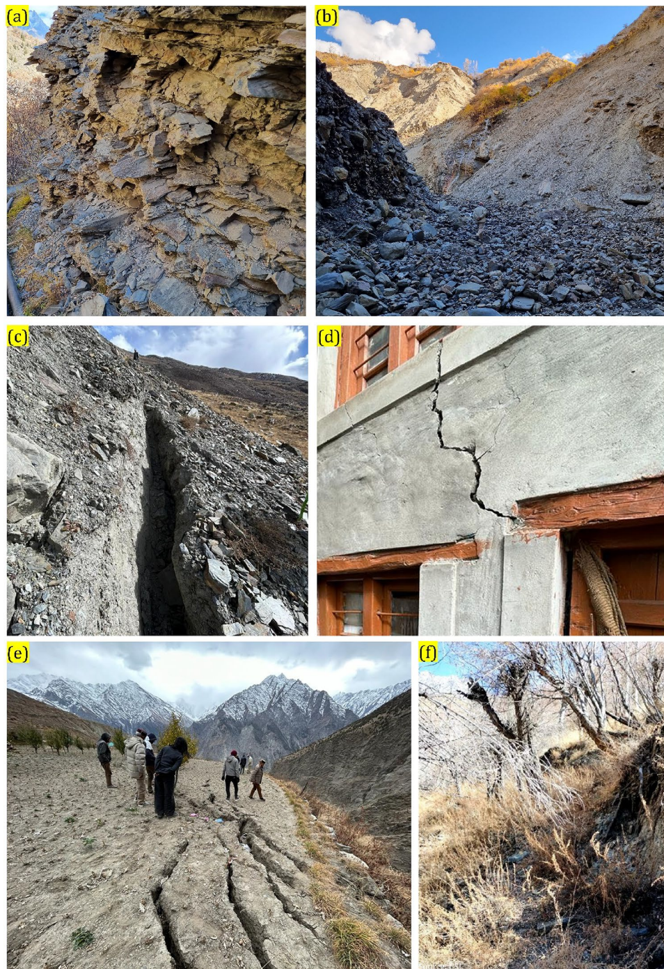
Fig. 9. Field photographs showing the local geology and cracks (a) Slate bed orientation along the slope gradient (b) Subsurface ice melt water stream (c) Crack present across the rock glacier in NE direction of the village (d) Vertical cracks on the wall of a house (e) NNE-SSW trending transverse cracks observed in agricultural field (f) Drunken tree present on the slope.
