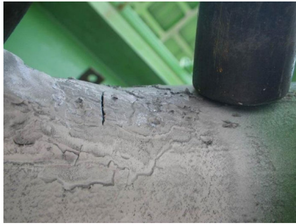
Fig. 10. Examples of damage after a failure of the carrying structure of discharge boom—cracks.
