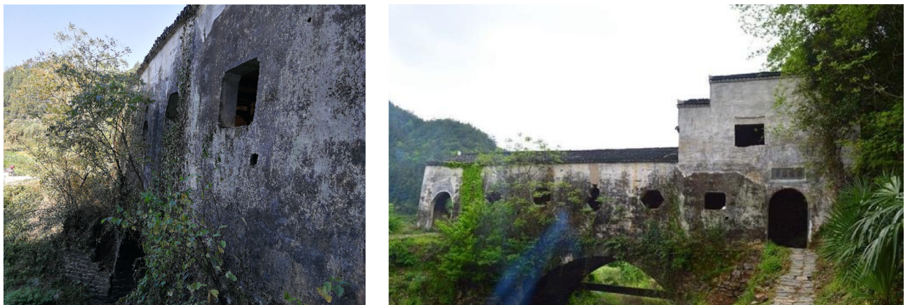
Fig. 2. (a) Current situation of weathering of Anfu Bridge wall; (b) Current situation of weathering on the facade of Anfu Bridge.
