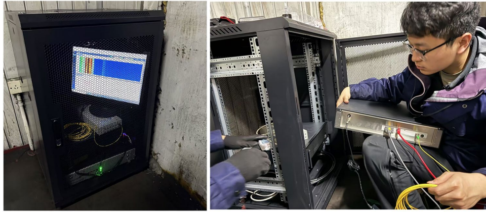
Fig. 17. Data acquisition setup for vibration measurement at the port conveyor belt system.
