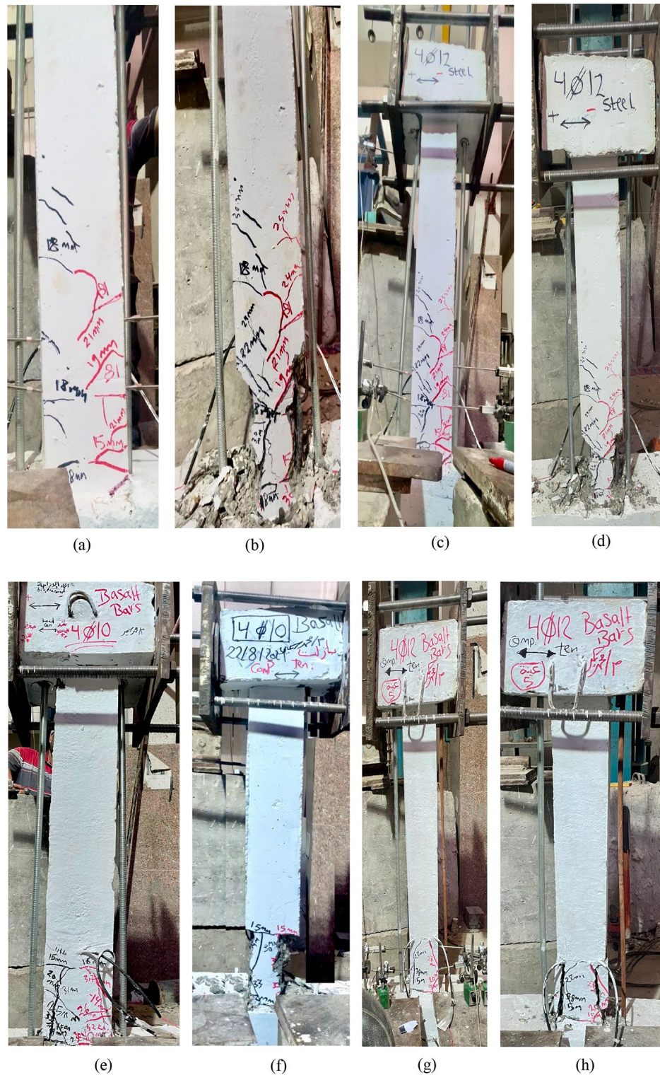
Fig. 6. Damage progression in UHPC column specimens under cyclic lateral loading: Steel-reinforced specimens: (a–d) Flexural crack initiation followed by concrete spalling and final failure in specimens reinforced with 4Ø10 mm and 4Ø12 mm steel bars. Basalt-reinforced specimens (4Ø10 mm): (e–h) Flexural crack initiation and subsequent concrete spalling leading to final failure in two specimens reinforced with 4Ø10 mm basalt bars. Basalt-reinforced specimens (4Ø12 mm): (i–l) Flexural crack initiation and concrete spalling leading to final failure in two specimens reinforced with 4Ø12 mm basalt bars.
