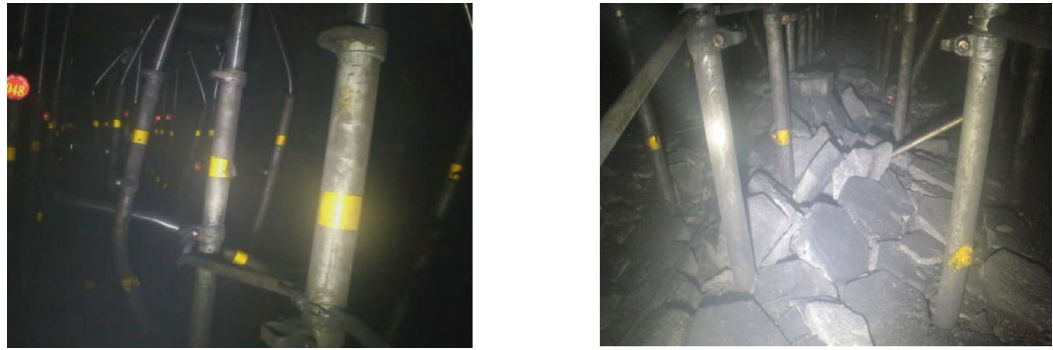
Fig. 1. Strong mine pressure behavior of 8105 working face.
