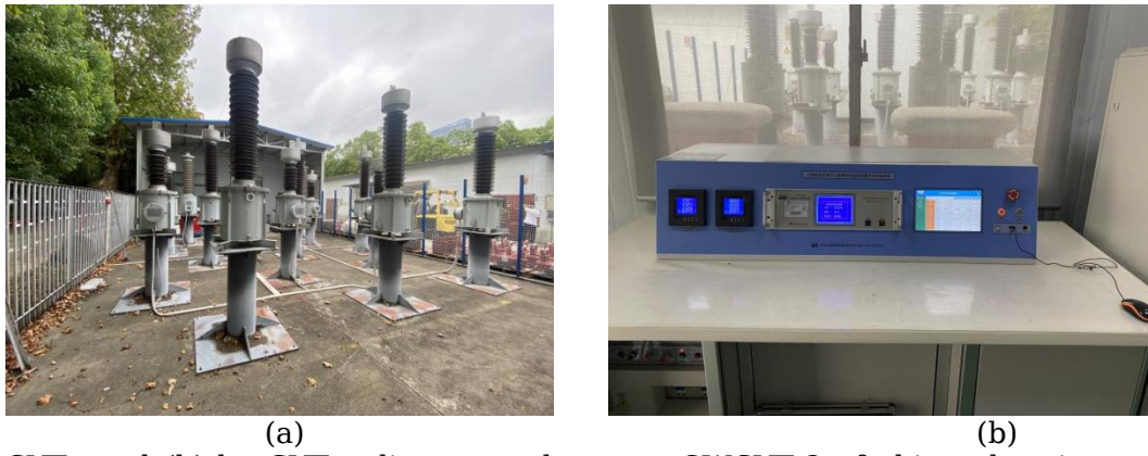
Fig. 2. (a) CVTs and (b) the CVT online control system SWCVT-3 of china electric power research institute.
