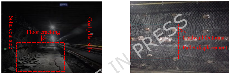
Figure 1. Tunnel deformation conditions
