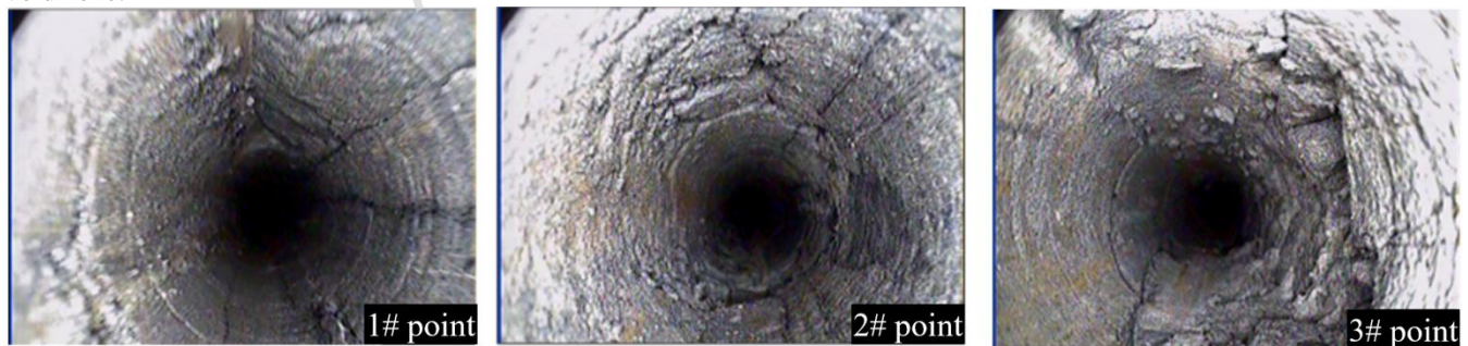
FIGURE 11. Characteristics of thick-hard roof fracture before and after fracturing.
