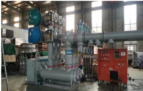
(a) 220 kV GIS disconnector
