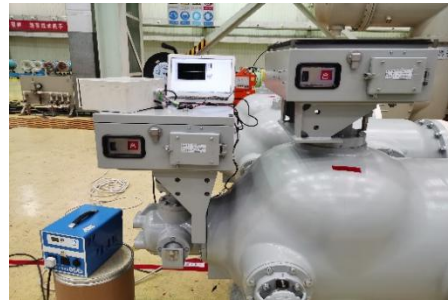
(b) 110 kV GIS disconnector
